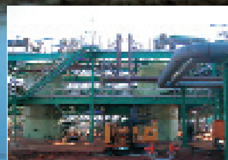
Top: The plant at night with HP compressor in the background. Centre: One of the dew point control units. Bottom: Inlet separators. Top right: View of HP compressors from the piperack.
