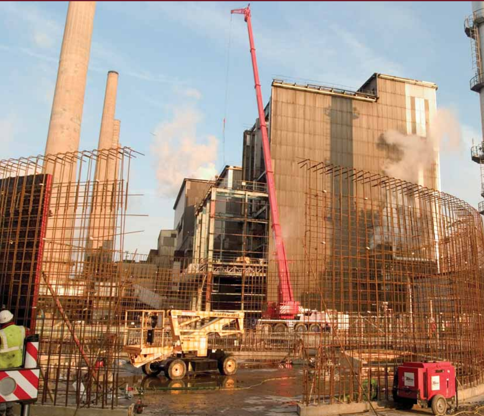
Reinforcement for a circular concrete wall which is the base of the fuel storage silo during site preparation.
