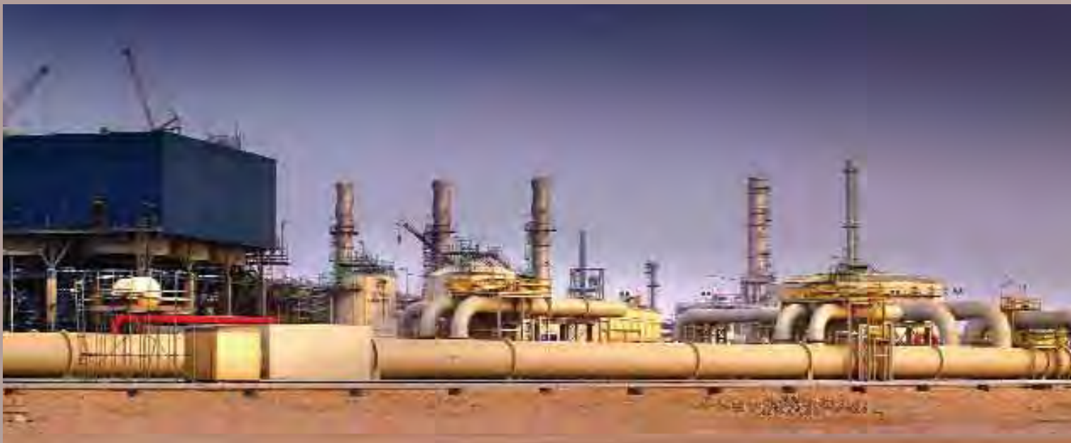
Top: One of the two cigar-shaped LTFT reactors, each weighing 2,100 tonnes, which lie at the heart of the ORYX GTL plant.
