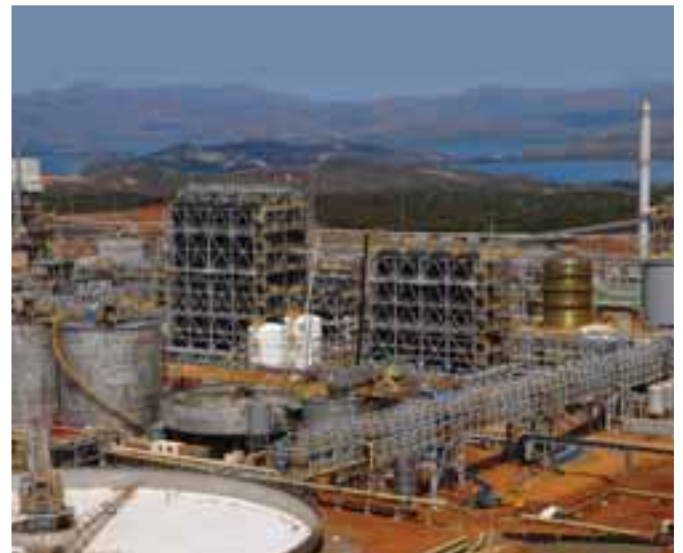
Images (clockwise): The Flamenco moored at the project jetty; the sulphuric acid plant; the team at site; overview of the plant and the primary solvent extraction area.
