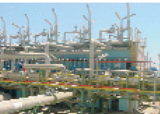
Palos de la Frontera. Top: Existing LNG tank and send-out pumps. Bottom: Seawater open rack vaporisers.
